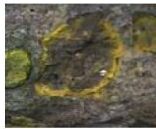
Concrete tested with yellow gel only showing beginning stages of ASR degradation.
