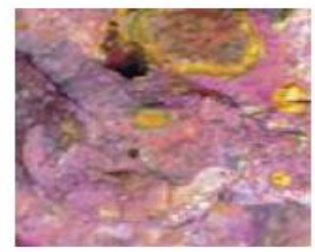
Concrete tested with pink and yellow gels showing both beginning and advanced stages of ASR.
