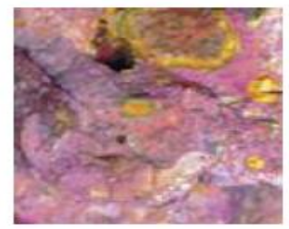
Concrete tested with pink and yellow gels showing both beginning and advanced stages of ASR.
